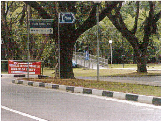
Road Kerbs Installed at Car Park C4, East Coast Park Service Road.
