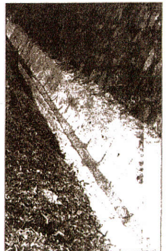
No different from a normal drain, this one, in Bukit Timah, was made with concrete waste.
